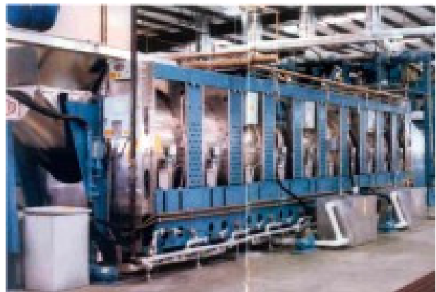
Chang-Gung Memorial Hospital- Tunnel washers
