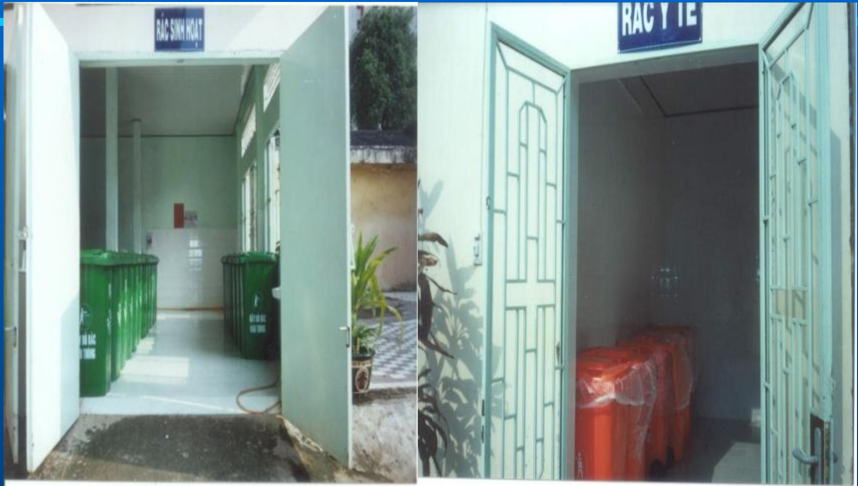
Medical waste storage
